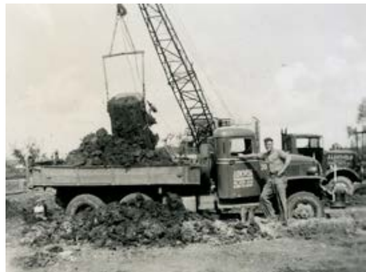
Earthmoving for the construction of a school. Dragline and GMC in the polder, 1955.
