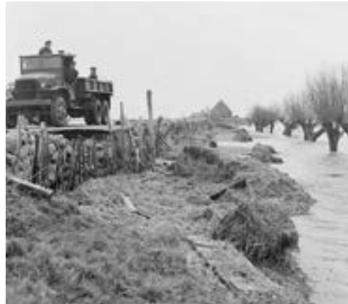
Relief work on a country road in a flooded area. Memory of the Netherlands collection.
